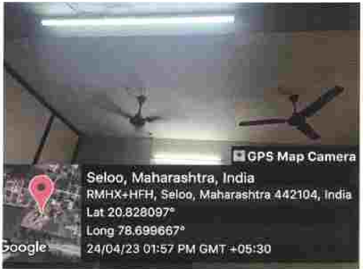
LED lights in Principal cabin
